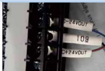
Visually confirm the wiring part
